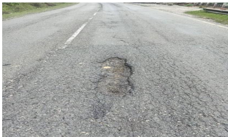
Gambar 2.23 Lubang ( Potholes ) (Sumber: Christady Hardiyatmo, 2015)
