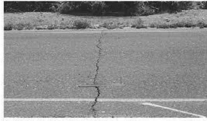
Gambar 2.11 Retak Melintang ( Transverse Cracks ) (Sumber: Christady Hardiyatmo, 2015)
