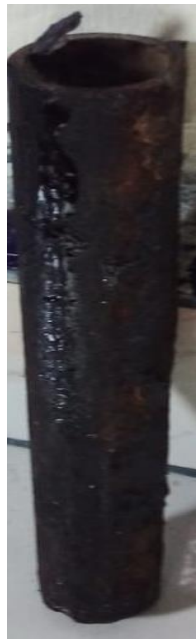
Gambar 1.1 Sampel pipa distribusi crude oil
