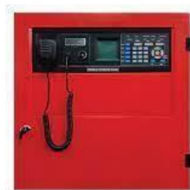
Gambar 2. 23 Fire Intercom Set
