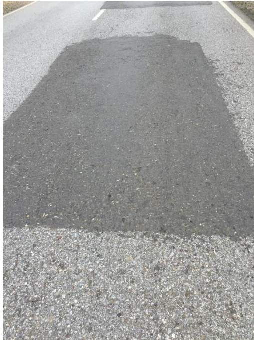
gambar 2. 13 Contoh Kerusakan Tambalan ( Patching end Utiliti Cut Patching )
