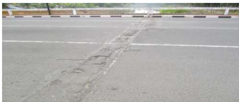
Gambar 2.7. Kerusakan Expansion Joint Jembatan Rasuna Said
