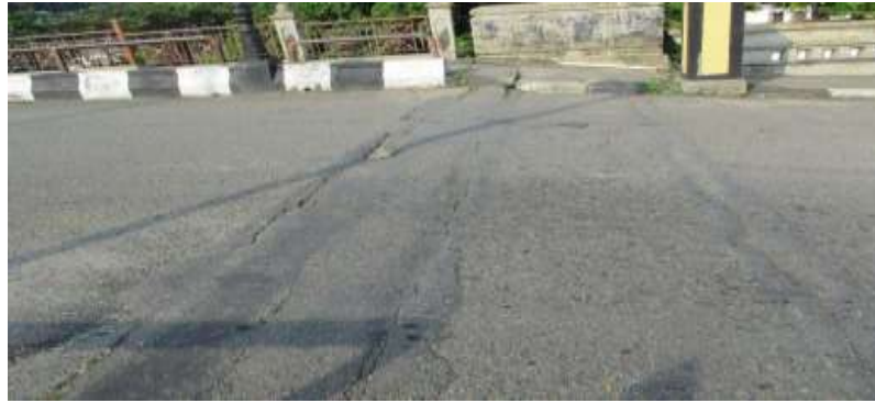
Gambar 2.8. Kerusakan Expansion Joint Jembatan Siti Nurbaya
