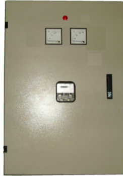
Gambar 3.8 Unit Panel Distribusi PLTS Terpusat.
