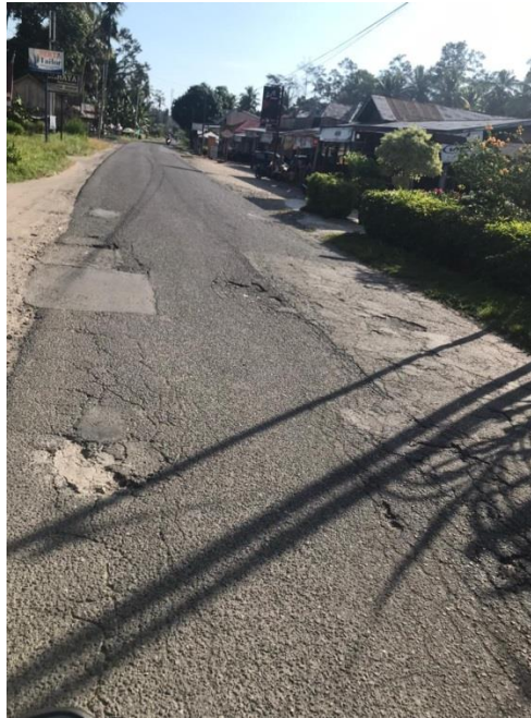
Gambar 1.4 Kondisi Jalan Raya Sicincin – Kurai Taji Pariaman km 62
