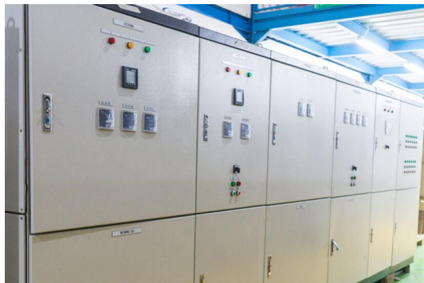
Gambar 2.12 Medium Voltage Main Distribution Panel
