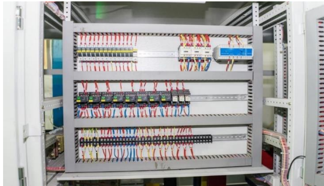
Gambar 2.13 Low Voltage Main Distribution Panel
