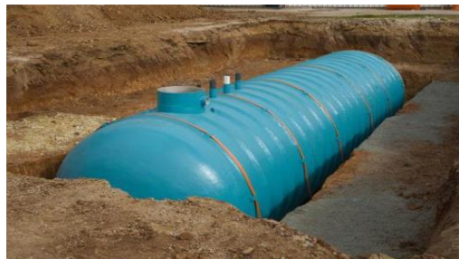
Gambar 2.41 Ground Water Tank
